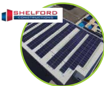
Shelford Construction 100kW System
